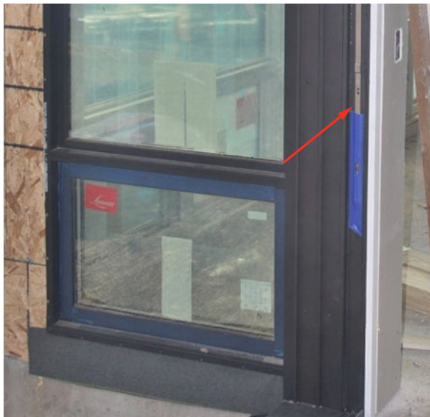
Interior track with spike plate
